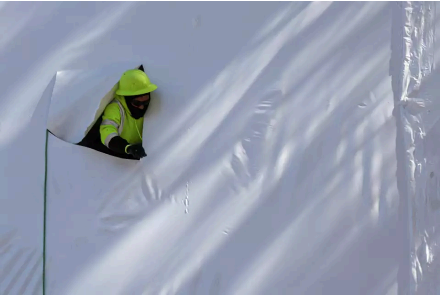
A construction worker sticks his head out from a plastic-wrapped Sugar Pine Village construction site in South Lake Tahoe. Tracy Barbutes/Special to the Chronicle
