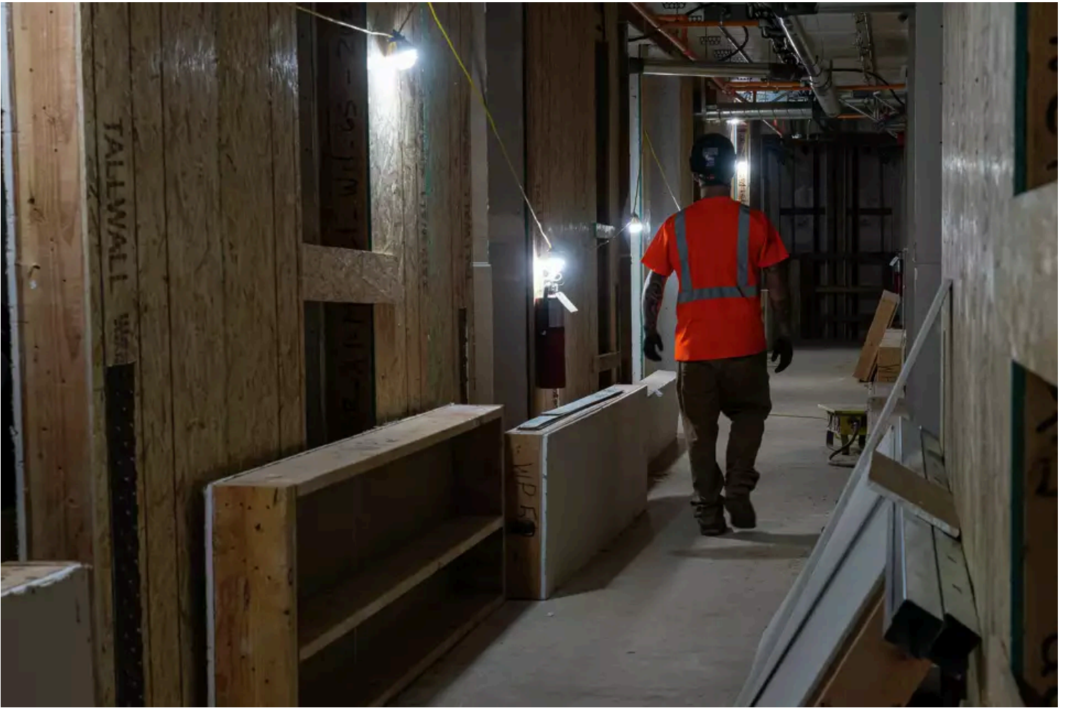
A construction worker walks along an inside corridor at a Sugar Pine Village construction site in South Lake Tahoe. Tracy Barbutes/Special to the Chronicle
