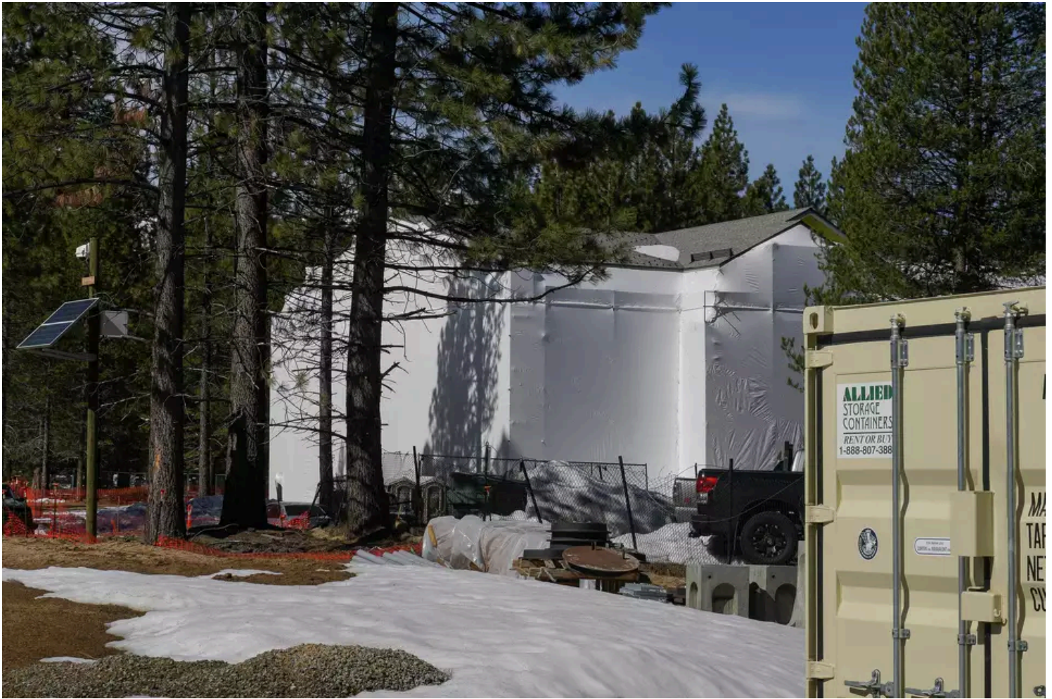
A Sugar Pine Village building, located off of Lake Tahoe Boulevard and Tata Lane, is wrapped in plastic during winter months. Tracy Barbutes/Special to the Chronicle
